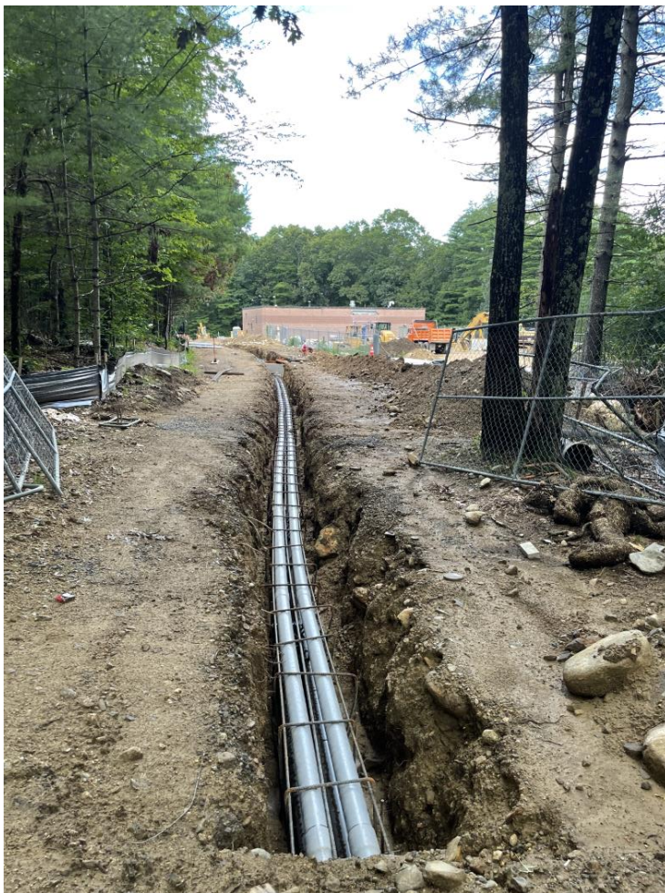
Looking north along the DPW access road behind Fowler School, electrical conduit lies in a trench extending to the treatment plant.
